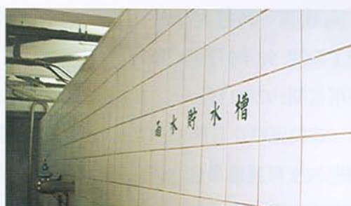
雨水配水槽(雨水及自來水自動切換)
